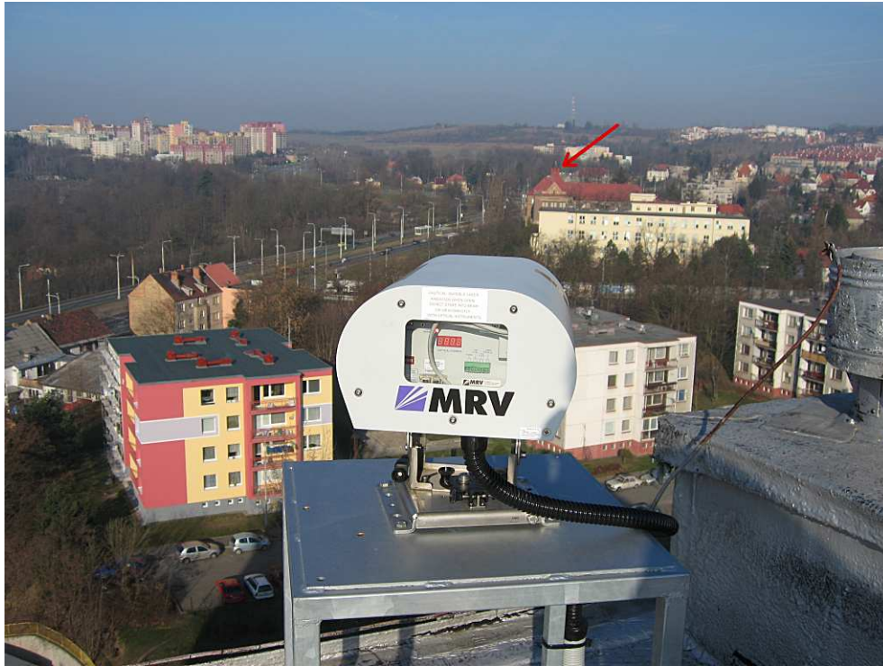
Figure 2: Full installation of the TereScope700/G laser link (the opposite end of the link is located at the top of the tower marked by a red arrow)
