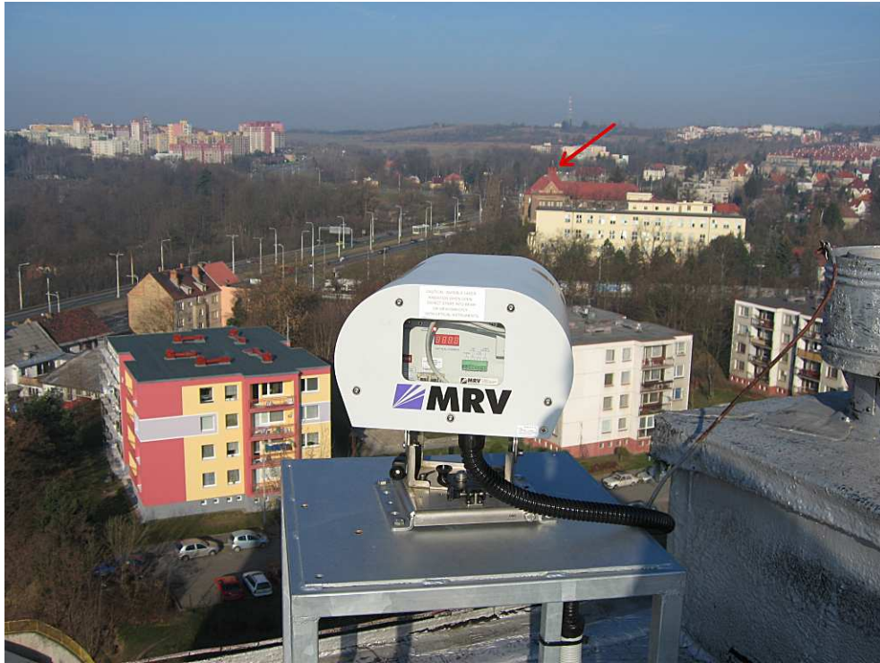
Figure 2: Full installation of the TereScope700/G laser link (the opposite end of the link is located at the top of the tower marked by a red arrow)
