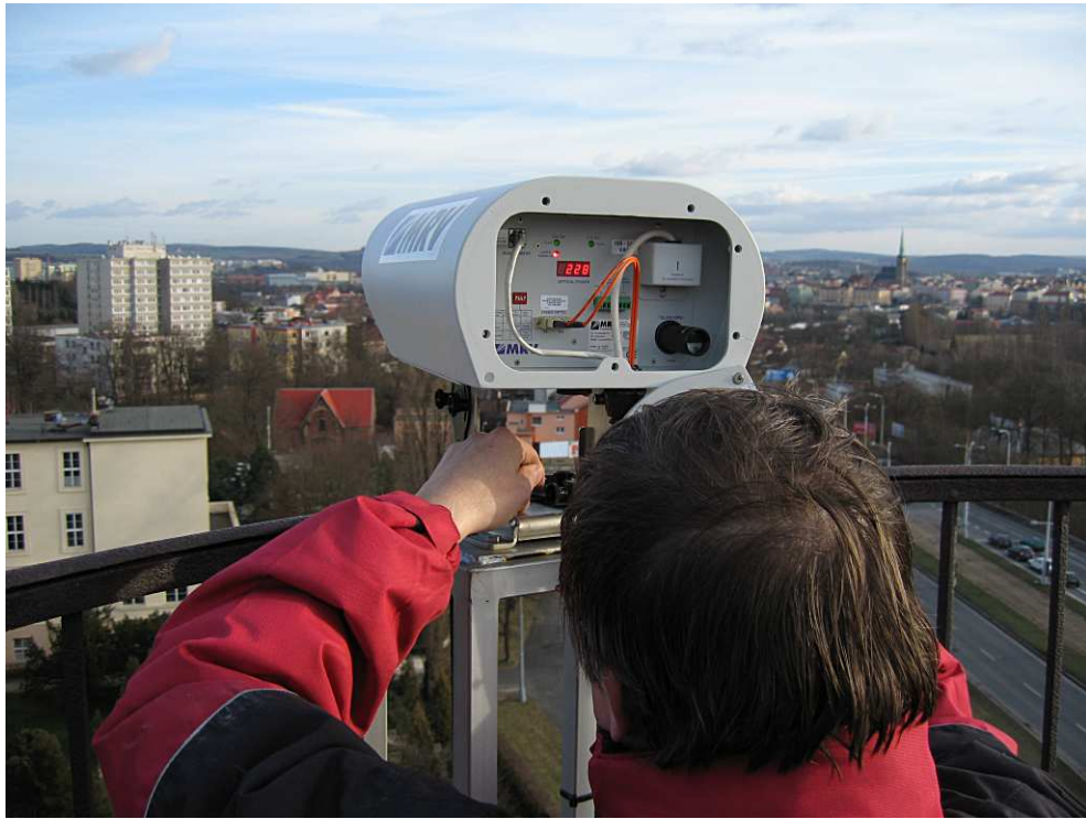
Figure 5: Installation and fine-tuning. The opposite end of the link is located on the roof of the block building in sight.
